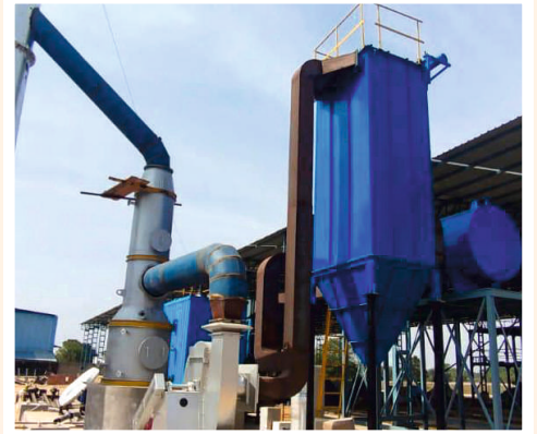
Bag Filter and Scrubber
