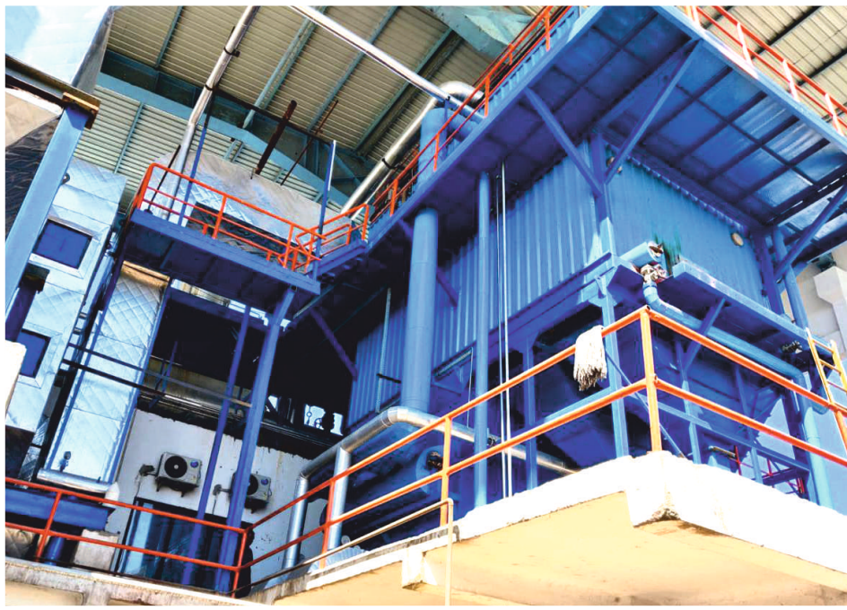
15 TPH Boiler (Isotex)
