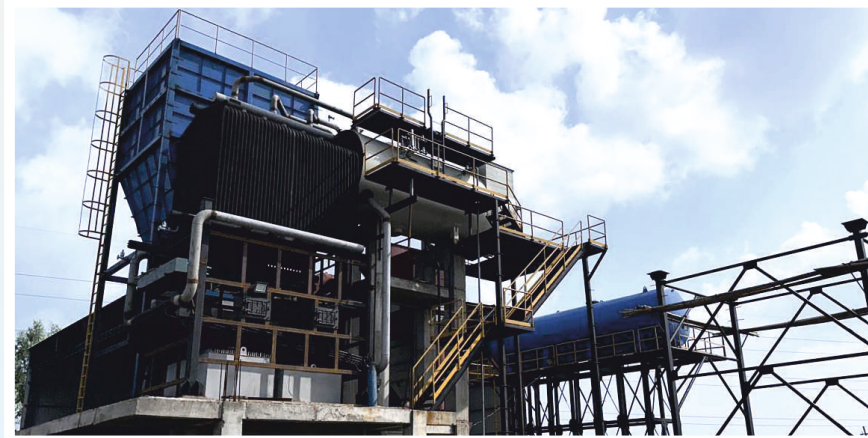
18 TPH Boiler (Cheema Boiler)
