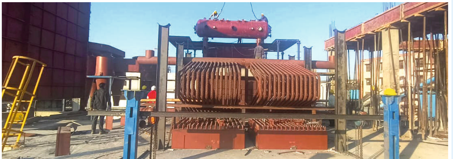
20 TPH Boiler IBL
