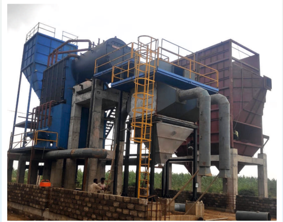
15 TPH Boiler Thermax
