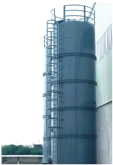
Oil Storage Tank
