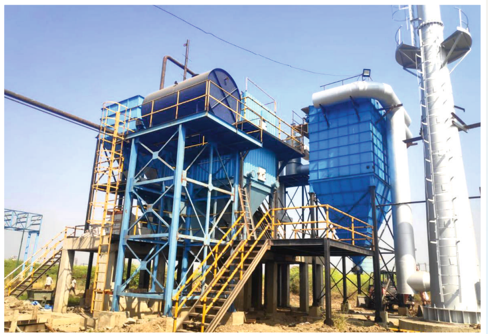
8 TPH Boiler (Isotex)
