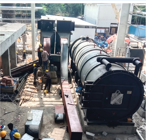
75 KL Gas Fire Thermopack (Isotex)
