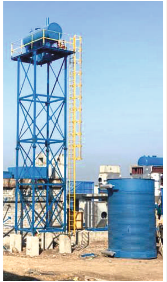
Oil Tank with Stucture
