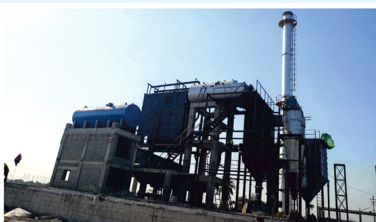
16 TPH Cheema Boiler
